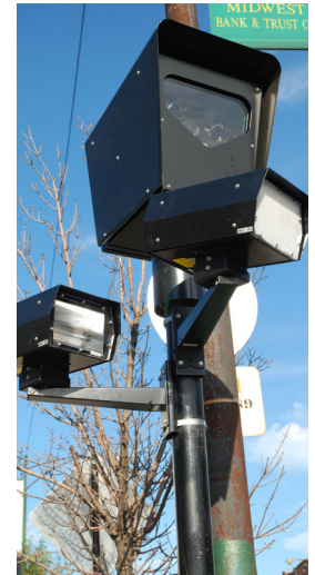
A red-light camera installed in Manchester, CT. Source: Mira Hartford, Flickr
