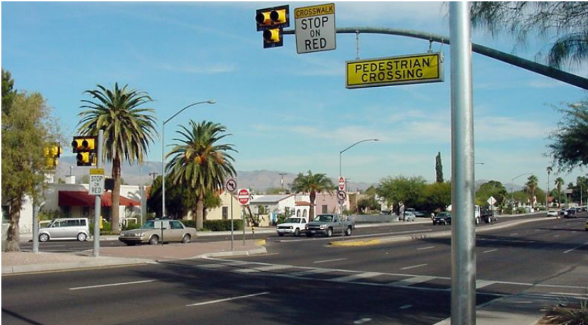
HAWK beacon on Third Street Bicycle Boulevard at Swan Road, Tucson, AZ. Source: Tucson Bicycle & Pedestrian Program, City of Tucson
